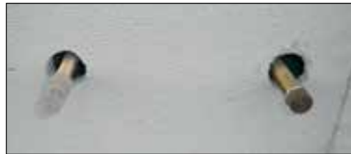
Figure 2.6.2 Neat finishes of installed services
